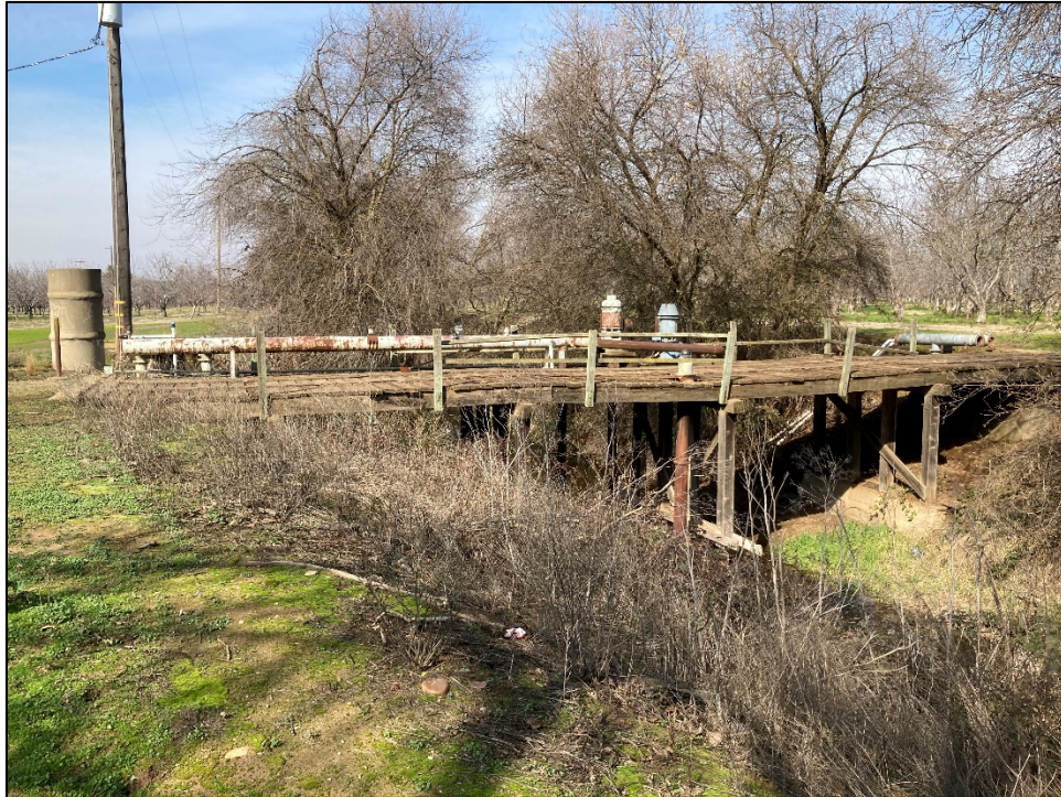
Photo 4. Representative photograph of the existing crossing. Photograph taken from the southeastern side of the bridge (January 2021). The new crossing will be constructed in the foreground of the existing bridge in this photograph.
