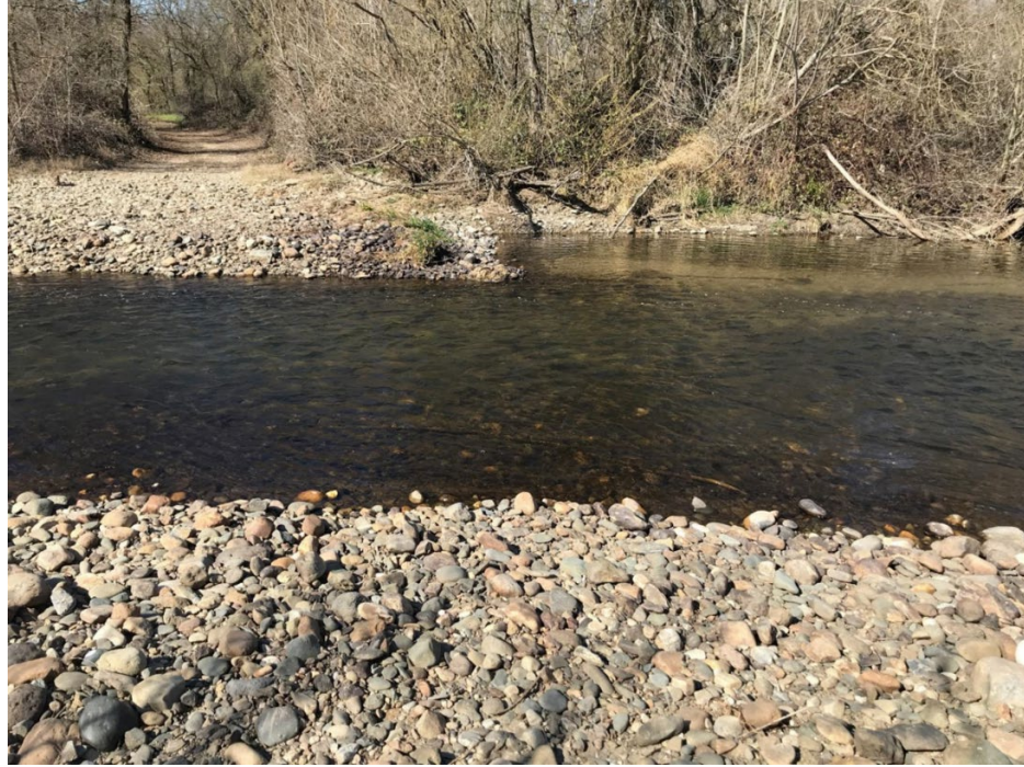
Figure 1. Washed out Low Water Crossing
