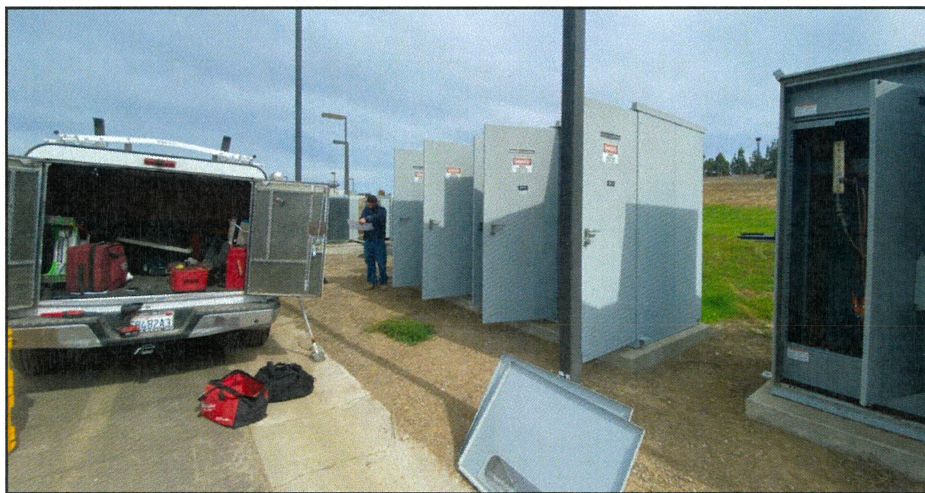
Figure 3. HSPS Switchboards Inspection
