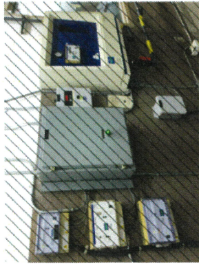
PHOTO - CHLORINATOR & INSTRUMENTATION IN CHLORINE GAS ROOM
