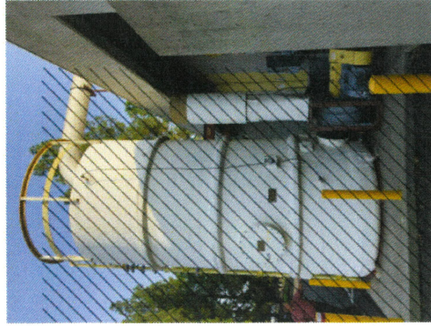
PHOTO - SCRUBBER (OUTSIDE)
