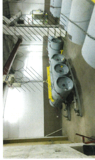
PHOTO - SCRUBBER (INSIDE CHLORINE GAS STORAGE ROOM)
