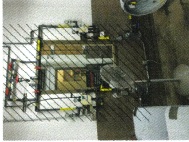
PHOTO - PIPING IN CHLORINE GAS STORAGE ROOM
