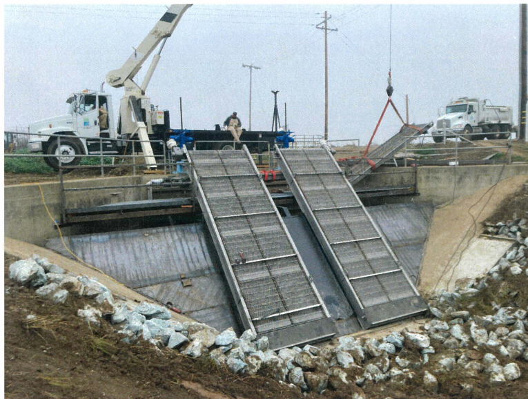
Figure 1. Funck Rd Traveling Water Screen and Conveyor System
