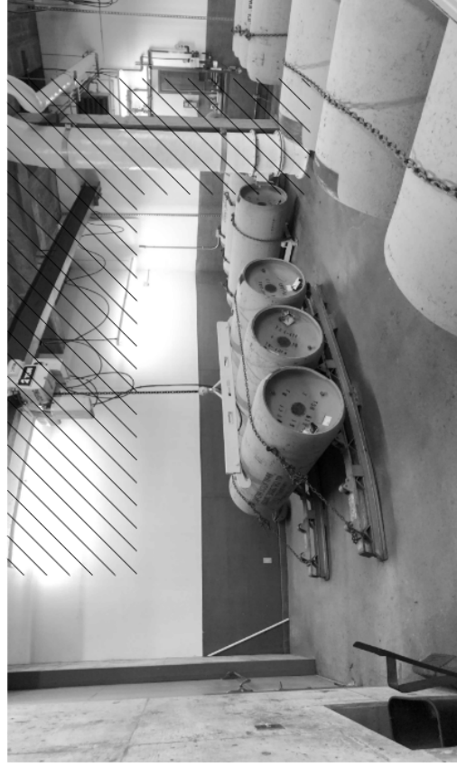
SCRUBBER (INSIDE CHLORINE GAS STORAGE ROOM)
